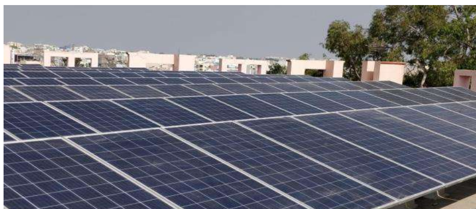
Figure 2.5: Grid Connected Solar PV systems (200 KV) installed on all buildings at ni-msme campus
